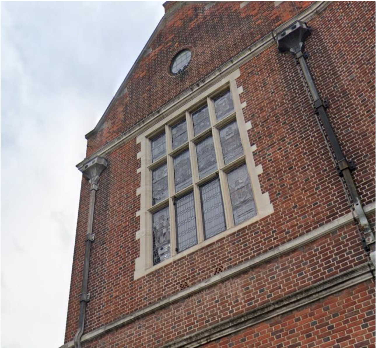
Photograph of the window concerned. Centre bottom two panels to have stained glass installed.
